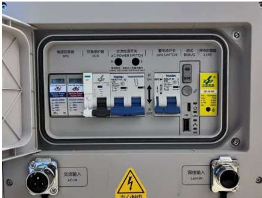
Figure 2-3 View of the electrical cabinet switches and ports
