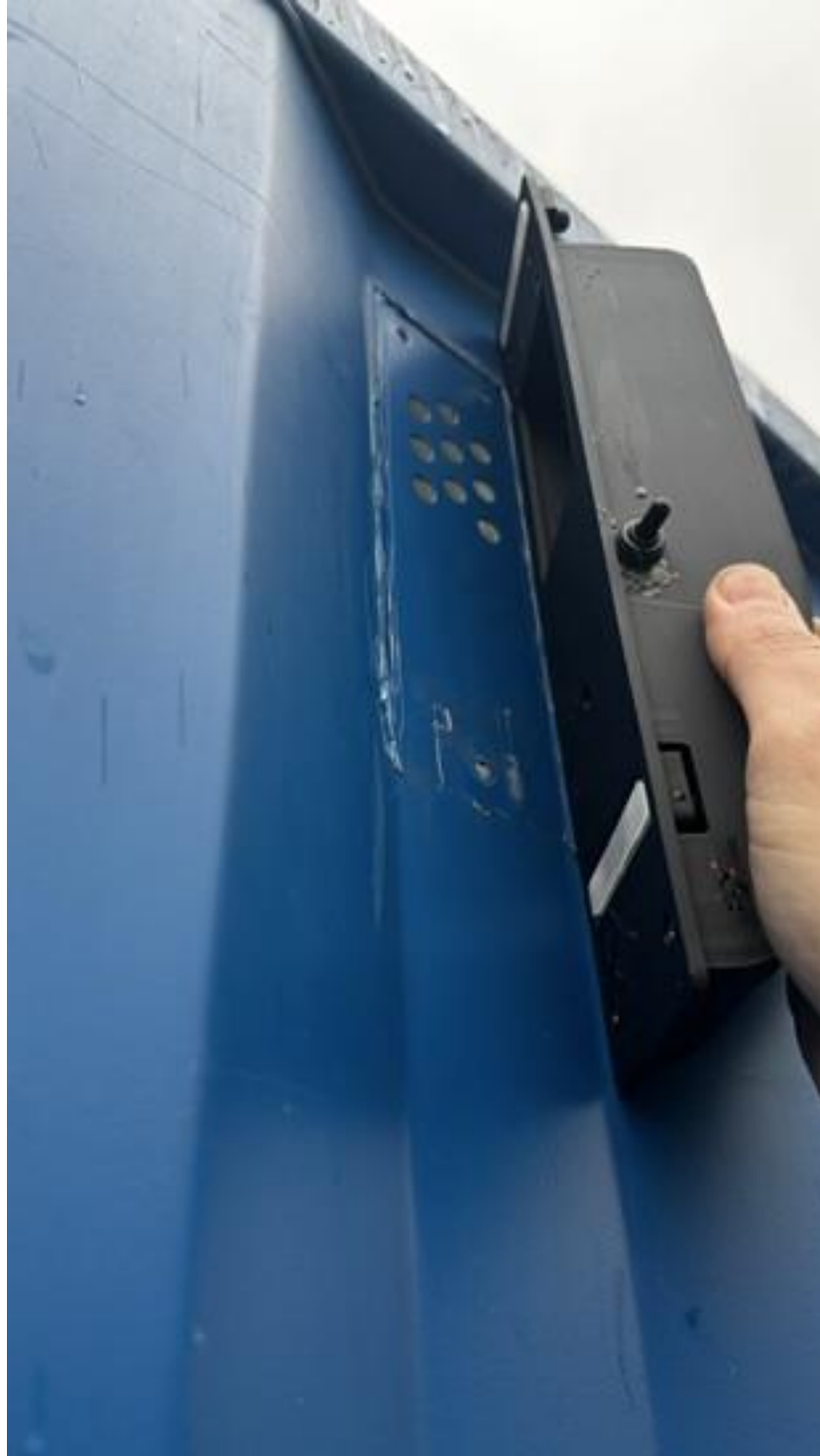
Figure 3 – Aligning OVERHEAT IoT sensor with the container air outlets
